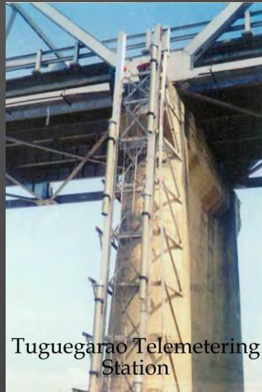
Tuguegarao Telemetering Station
