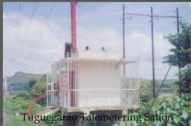
Cagayan Repeater Station
